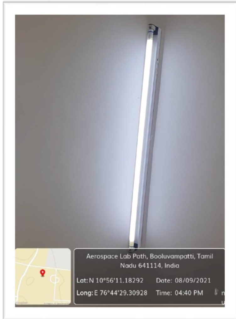
Fig 9. LED Tube Lights in the Classrooms.
