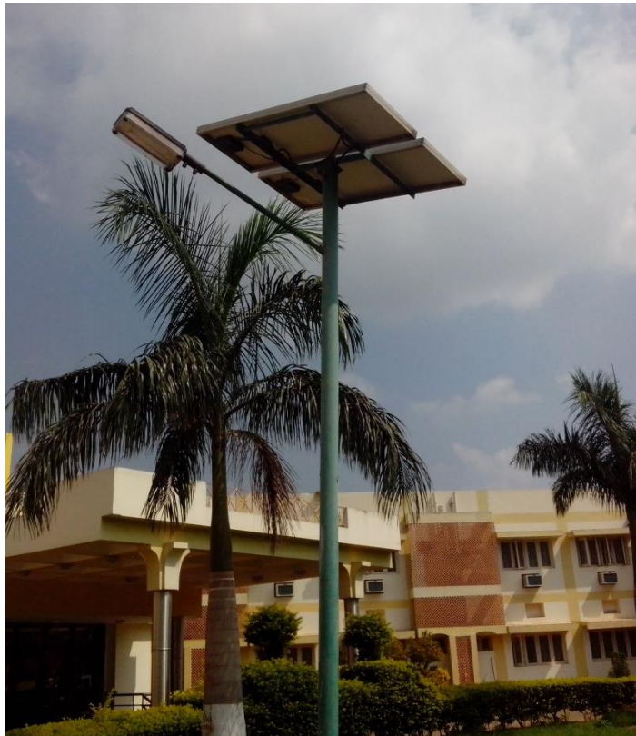
Fig 1. Solar based Street Light
